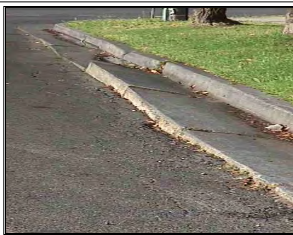
Condition 9 Extreme movement and lack of Function
