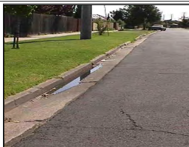
Condition 8 Large movement and holding of water
