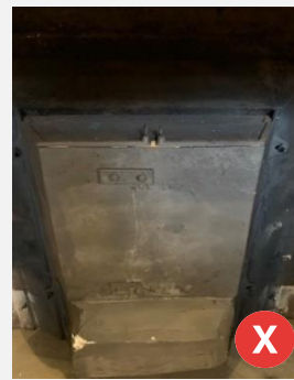
Figure 6: Interwar period fireplace which fully seals – rear view
